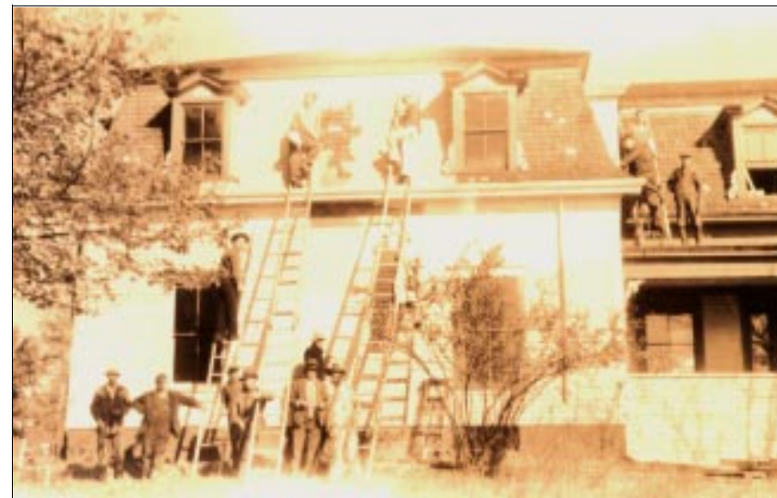
Work crew converting the old Summit House to the Doctor's House. [Note “summer kitchen still on rear before it was moved to the Porters]
