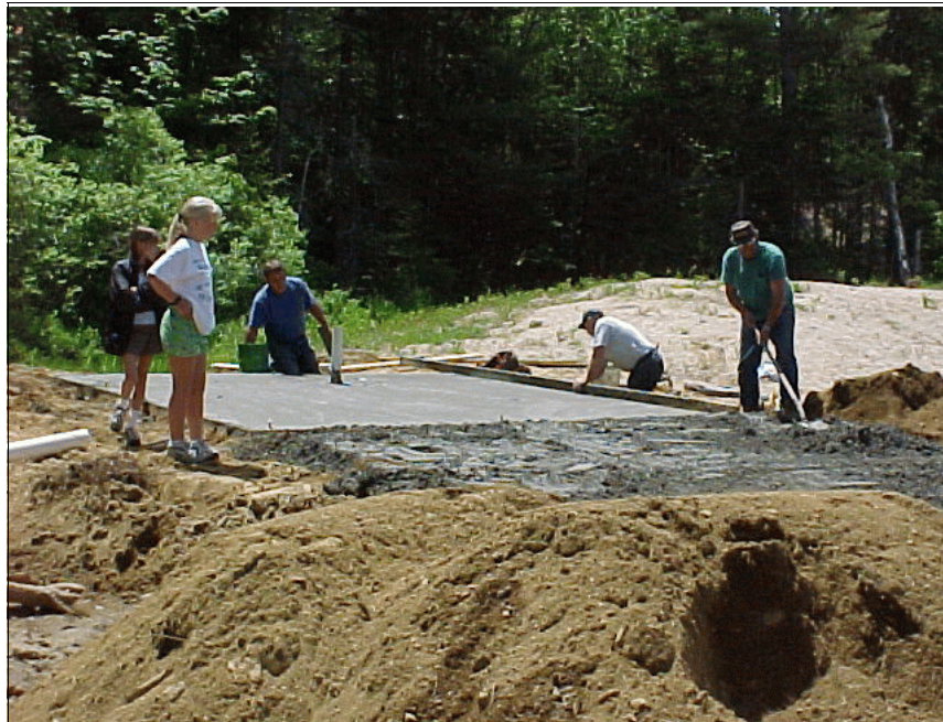
Public rest room takes shape in back of the Historical Society building
